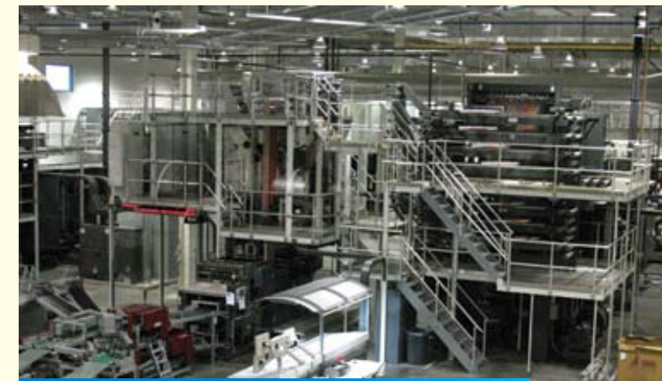
In the press hall, two Goss Sunday 4000 web presses print non-stop with a plate change every 12 minutes on alternating sets of cylinders.
